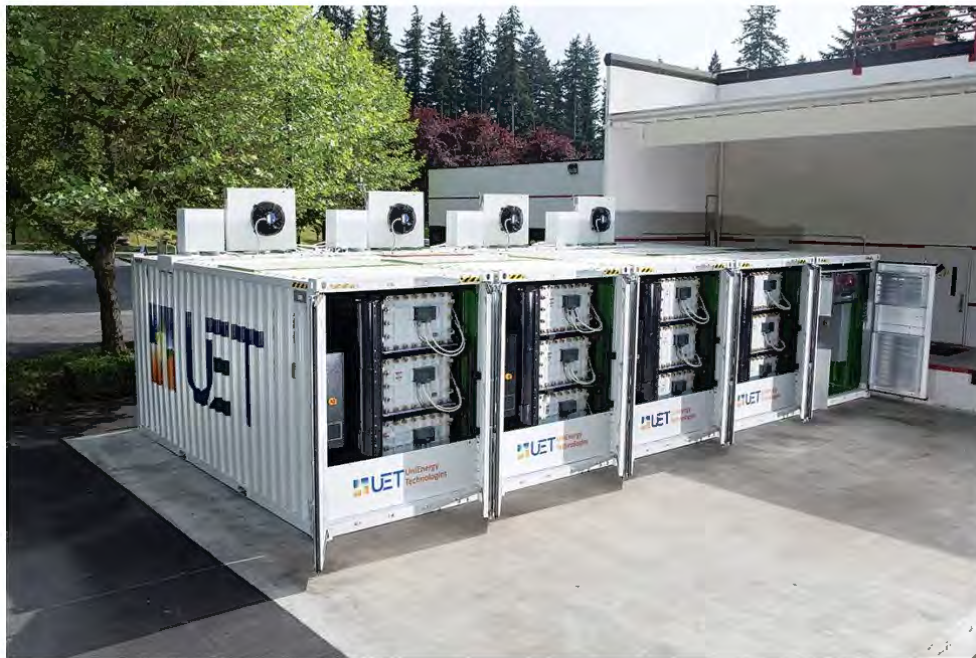
Figure 8: Photo of a Vanadium redox-flow battery. UniEnergy Technologies Source: IEEE Spectrum
